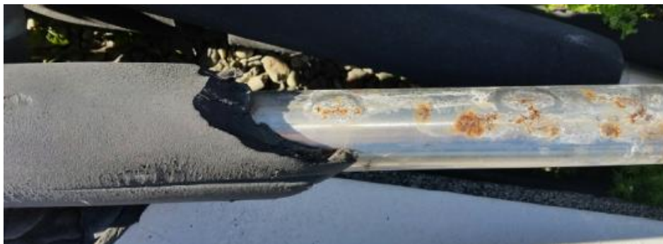
Photo: Venison Processing Plant, NZ – 2015 (SCC and localised corrosion induced by 'standard' lagging).
